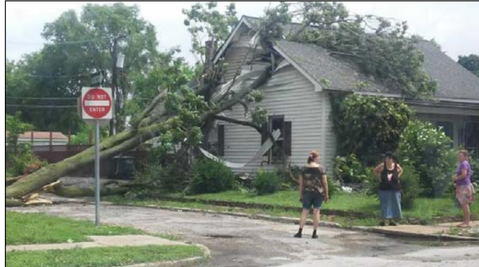
Damage sustained in Danville during the June 7, 2015 thunderstorm with damaging winds.
