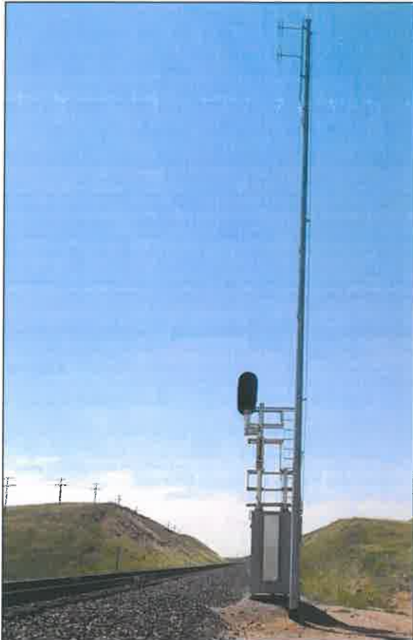
Standard pole and equipment bungalow example for Union Pacific Railroad's PTC poles.
